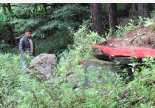
Damaged water tank.
